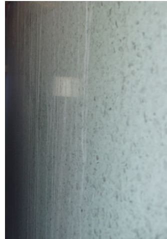
FIGURE 1 Example of a slab that was etched from condensation
